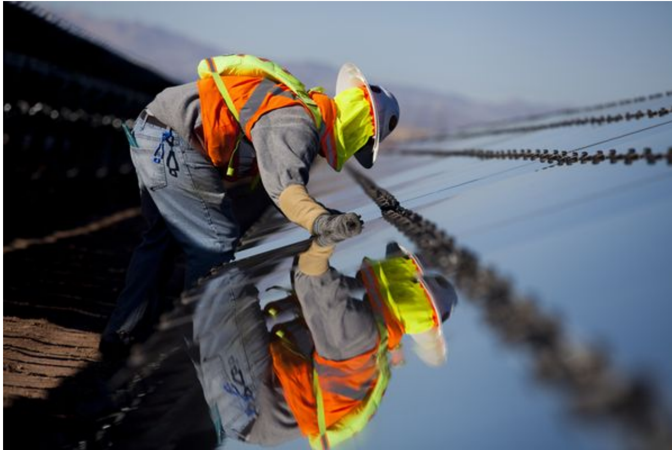
First Solar panel installation in California. The company is among those in Active Solar's $290 million portfolio. Photographer: Sam Hodgson/Bloomberg
